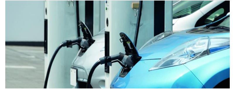
Secure EV charging Integrity & payment
